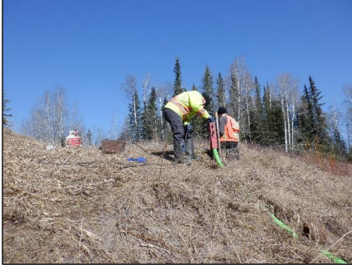
a. Steaming out the inlet hose for sensor installation for spring melt, April 18, 2024
